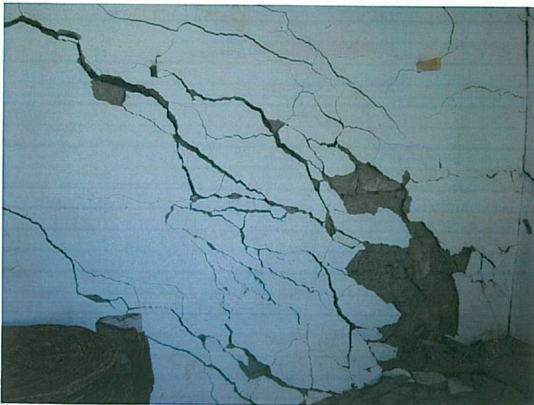
Figure 3.5: House damaged due to cracks on terraces
