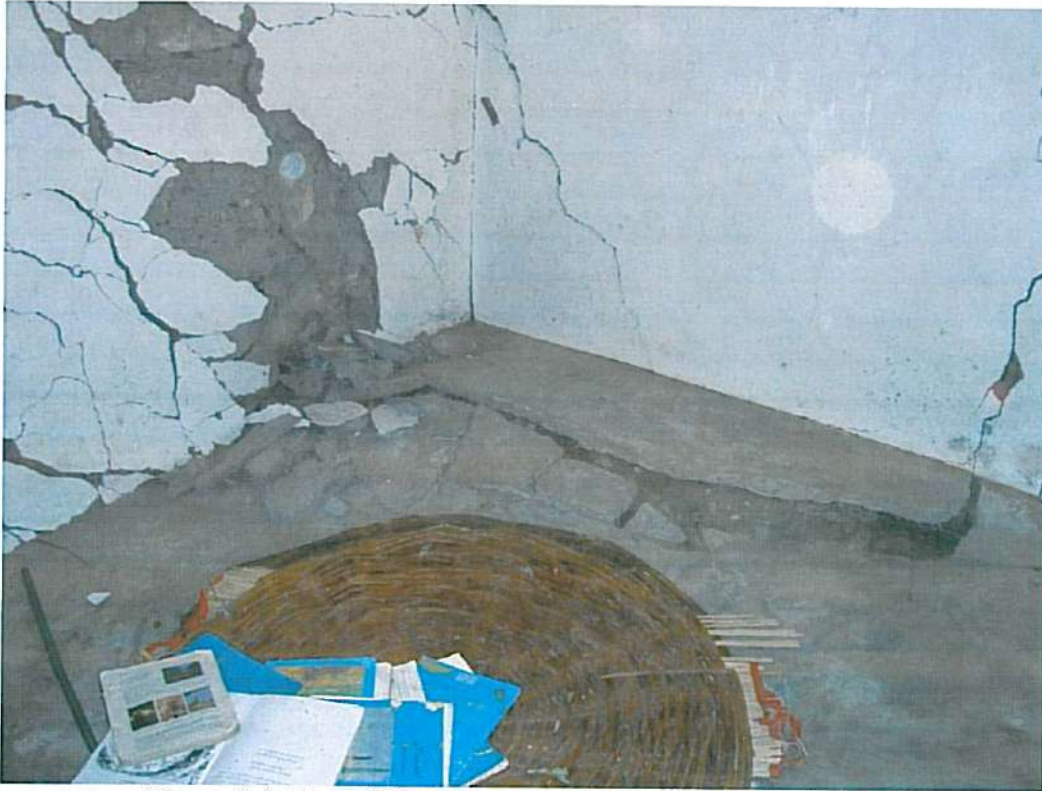
Figure 3.4: Slope failure at terraces have damaged the house
