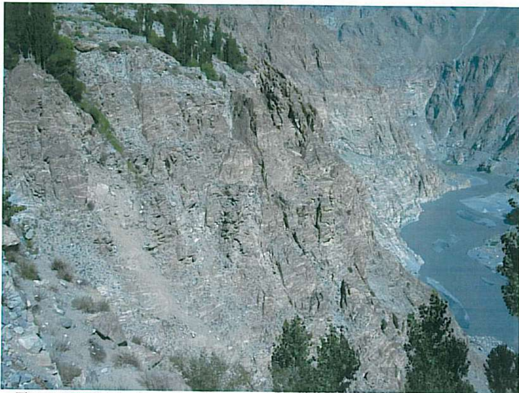
Figure 3.7: Highly sheared and fractured bedrock forming the toe of Atta Abad
